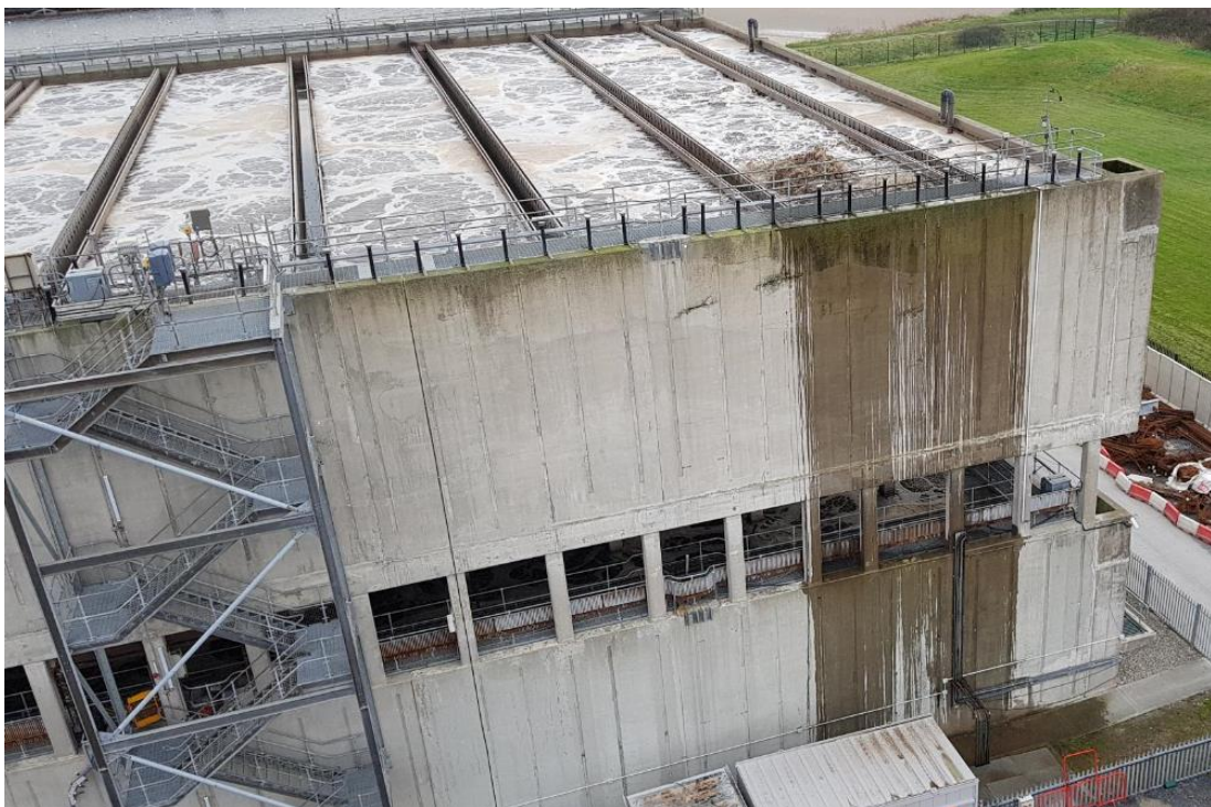
Fig 3.2 Overflow Incident – 9.30am - 23 rd February
